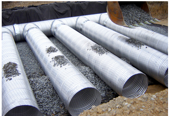
Stormwater management at Mantua
