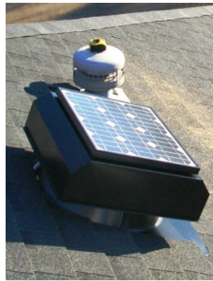
Solar photo-voltaic panel
