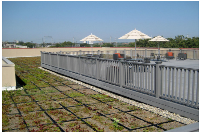
Green roof and roof-top patio at Warnock Senior Housing
